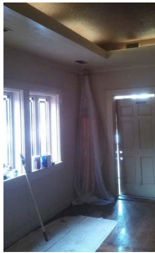
Some of the repaired soffit, new wall paint, old door from parking lot to Chapel interior.
