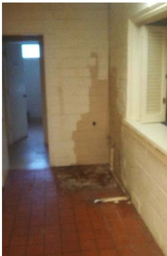
The corner of the kitchen from which the Coke machine and counter have been removed.
